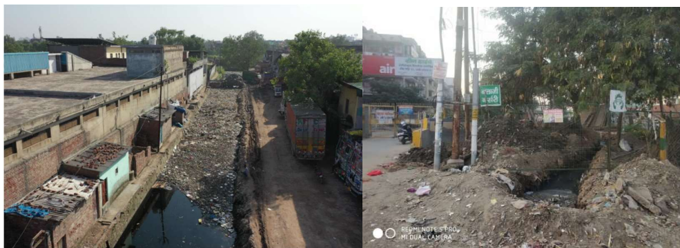
Figure 6. Unauthorized connections and structural damage.
