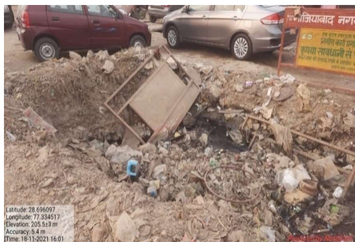
Figure 8. Bhopura pipe burst location
